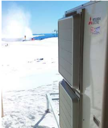
Zubadan Series installed at The Lodge – Ruapehu Ski Club .
